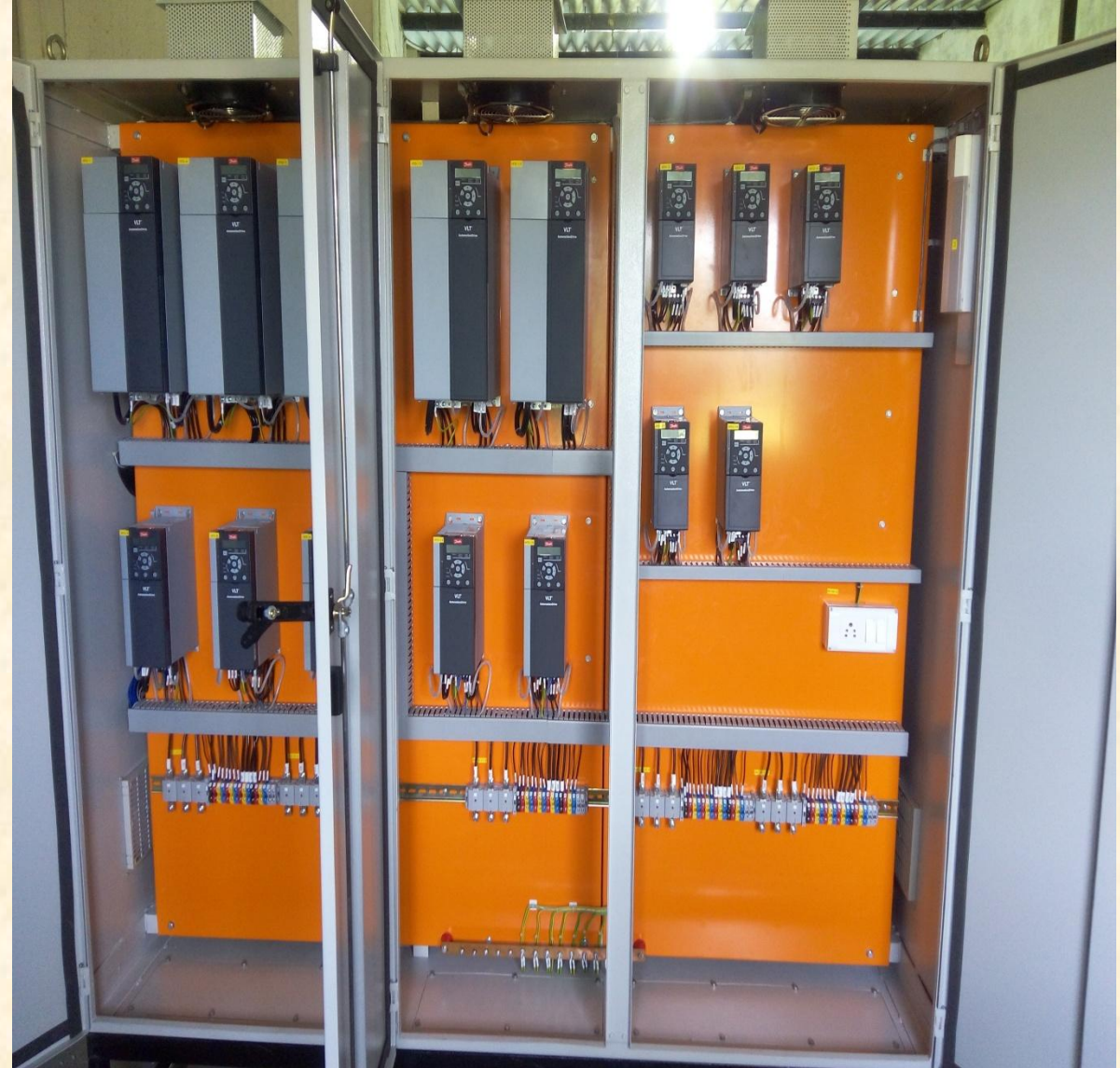
INNER VIEW OF VFD PANEL
