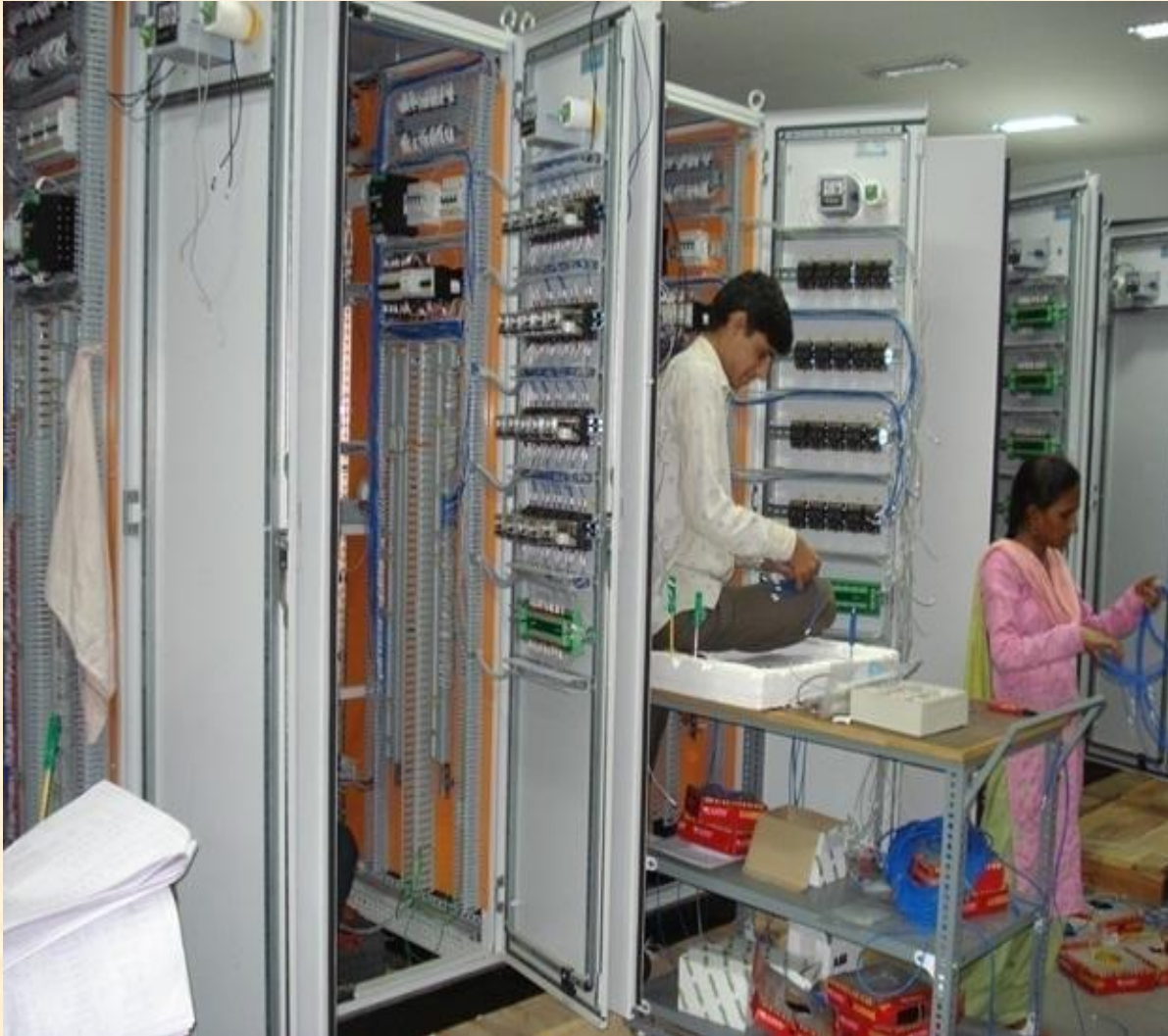
WORKMENSHP IN RELAY METERING PANEL
