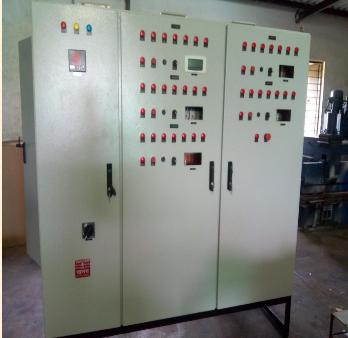
VFD PANEL FRONT SIDE
