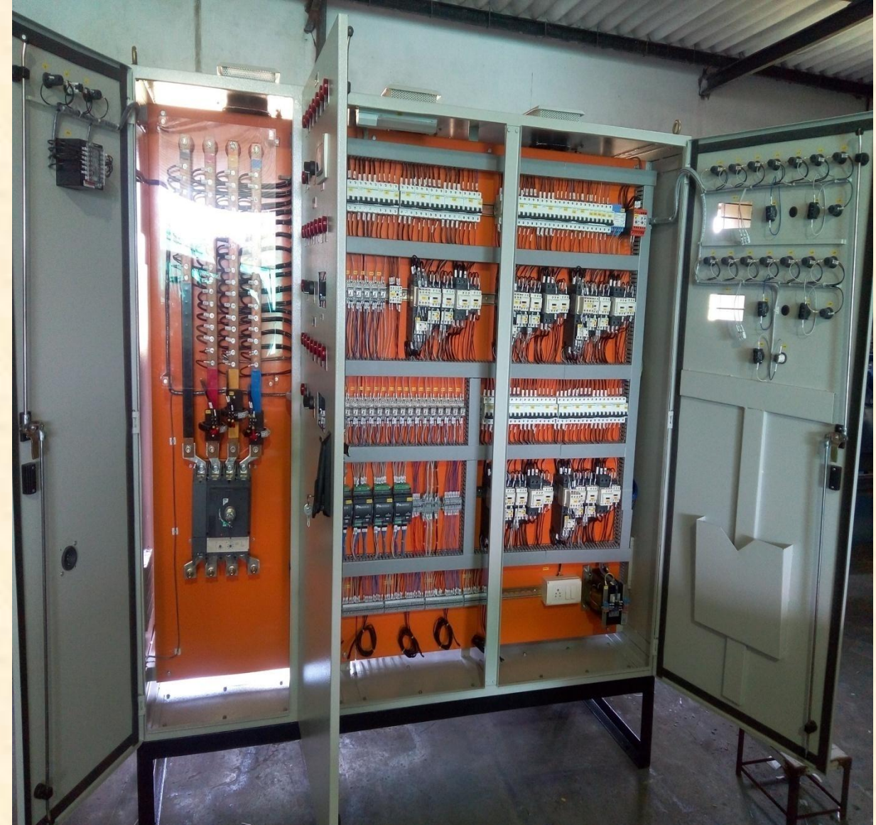
VFD PANEL WIRING VIEW
