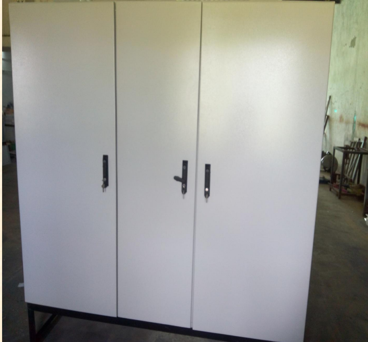
BACK SIDE OF VFD PANEL
